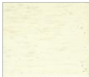
WITHOUT Sealing Primer, yellow discolouration appears on the surface.
